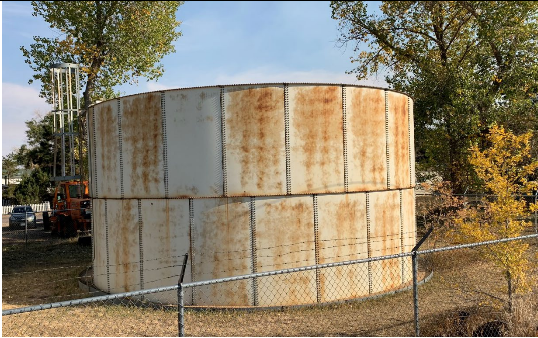
Figure 2. Tank Used for Disinfection Requirements. Note the Condition of Rust.
